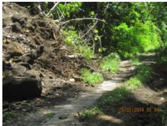
Figure 40 Need for protection of slopes against erosion
