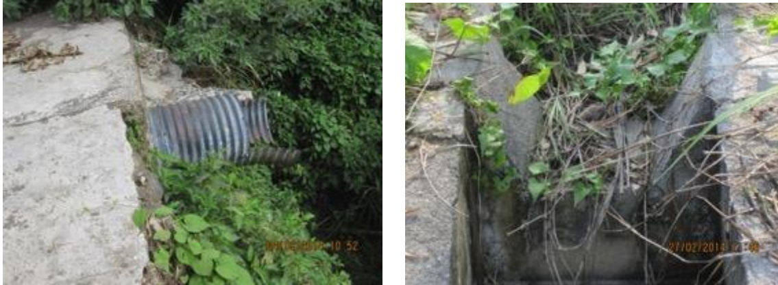
Figure 30 Cross drainage poorly maintained (Tanna roads)
