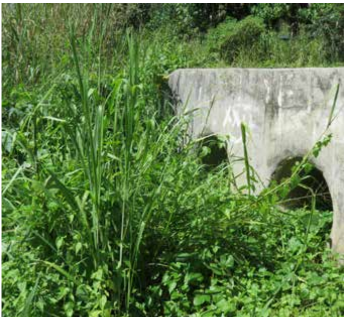
Over grown, blocked culvert, South East Coast Road, Santo
