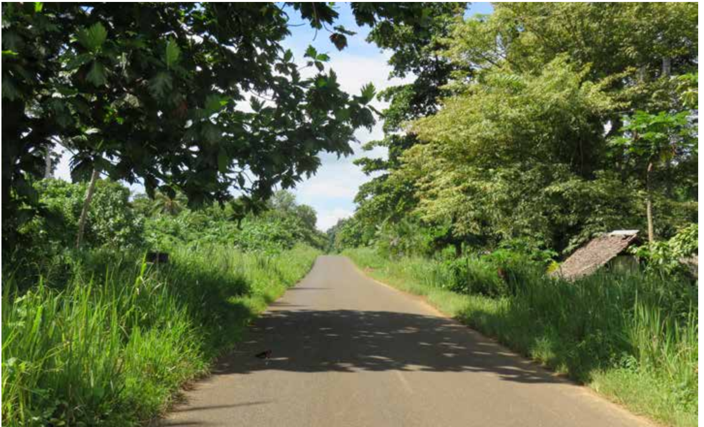
Overgrown grass and branches overhanging side drain and road, South East Coast Road, Santo
