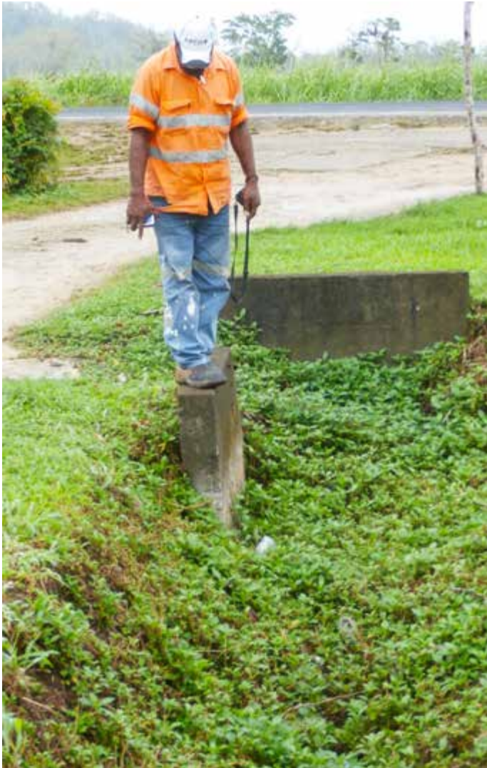
Over grown wing-wall, Efate Ring Road
