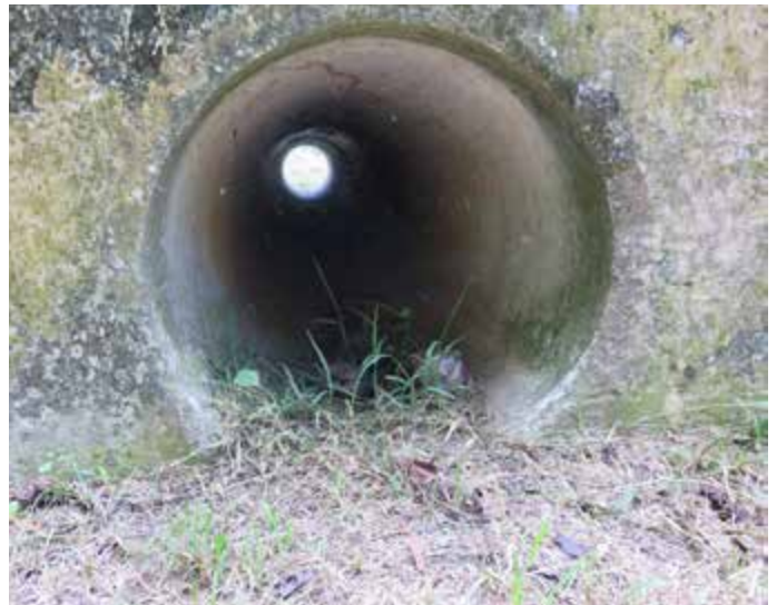
Remove vegetation and flood debris from culvert inlets and outlets, South East Coast Road, Santo
