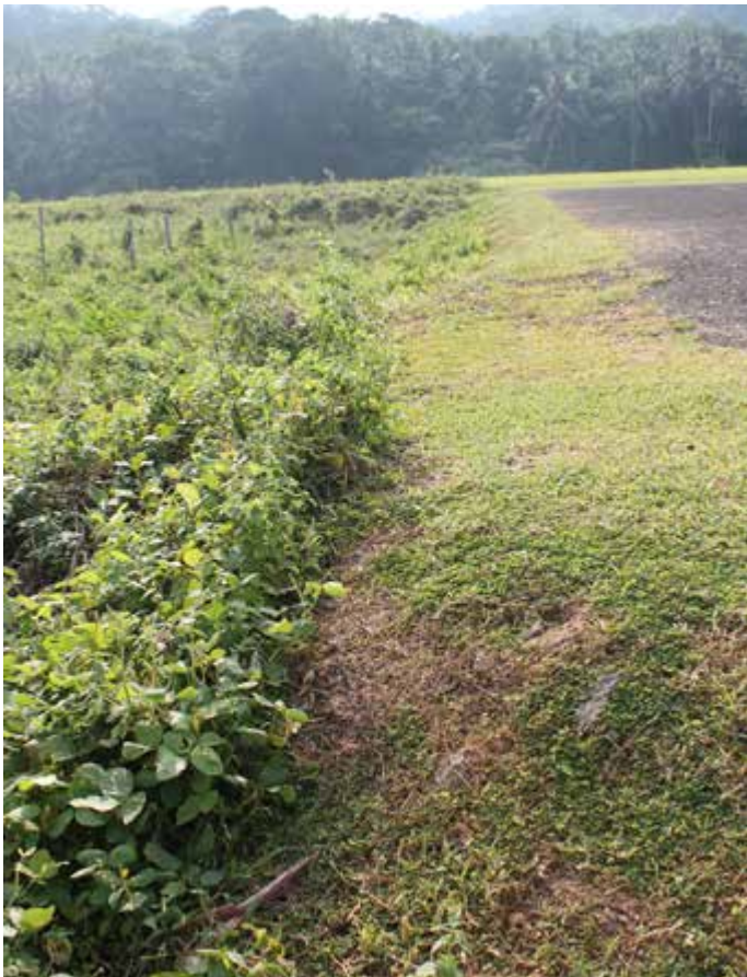
Side drain and fence line, Longana Airport, Ambae
