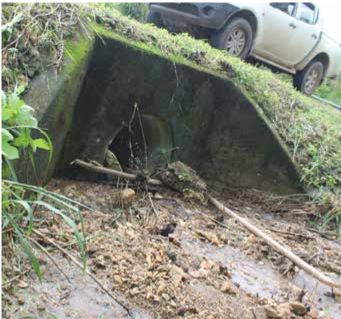
Blocked culvert, Efate Ring Road
