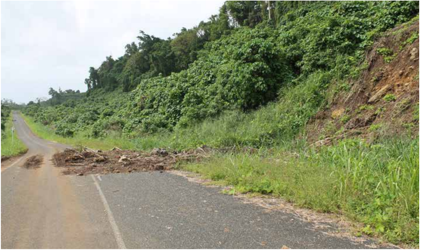
Landslide at Forari, Efate Ring Road
