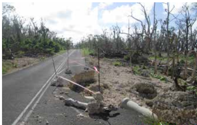
Storm surge damage during Tropical Cyclone Pam in 2015, Epau, Efate Ring Road
