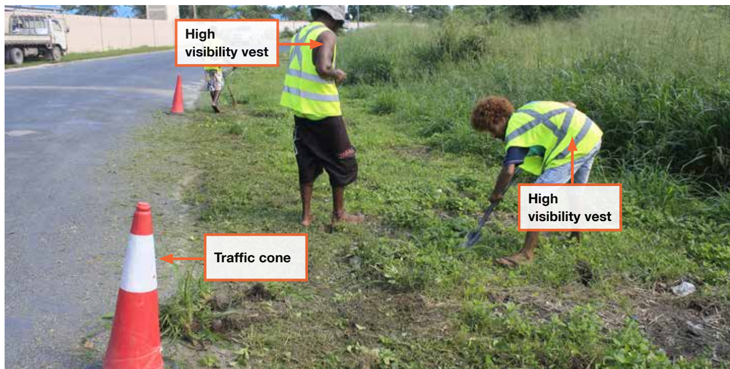
CBC workers wearing high visibility vest and traffic cones for traffic controls
