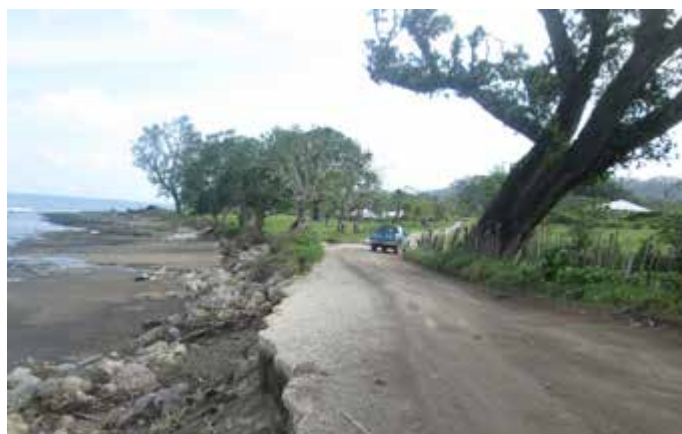
Storm surge damage, Devils Point Road, Efate
